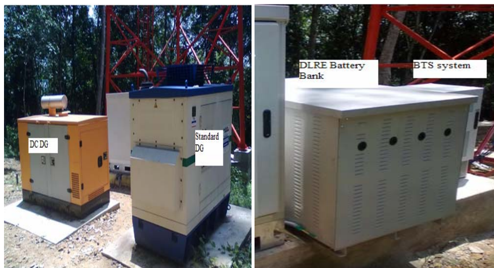
Figure 11: Field testing of BTS power system using HybridGEN DC VSDG
