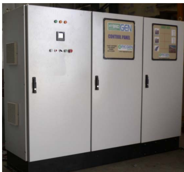
Figure 4b: Power conditioning unit
