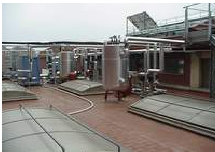
Figure 6: Solar AC Plant built by Siemens in Spain
