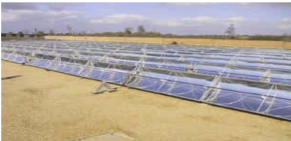
Figure 5: Use of Solar Heat (1.33 MW) in Industrial Process in El-Nasr City, Egypt
